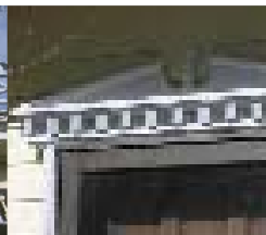
Broken pediment above door
