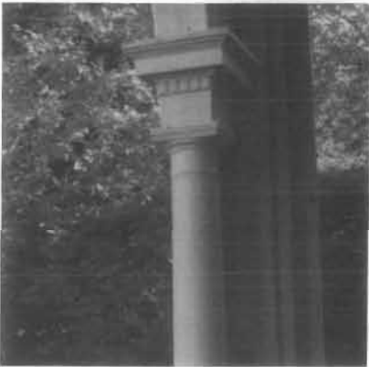
To replace deteriorated portions of the column, strips of new wood were milled to conform to the shape and appearance of the old column framework, glued in place, then back-primed and painted.
