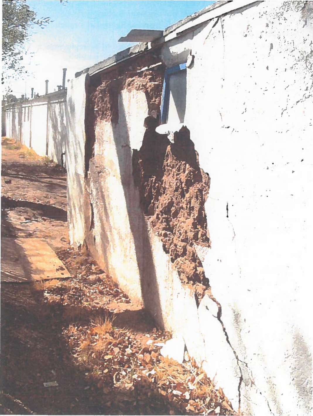
Figure 15 Wall Failure at Southeast Building Cluster
