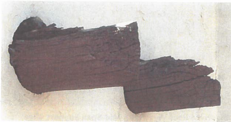
Figure 22 Dry Rot Viga Ends
