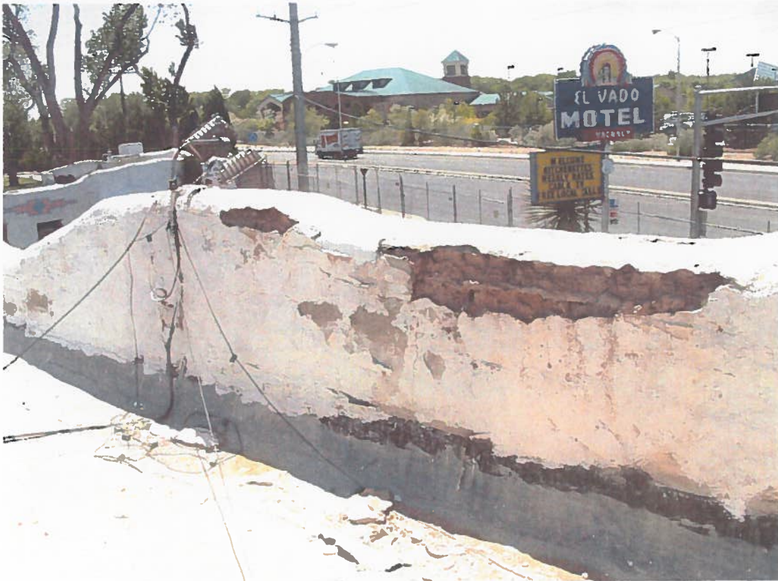
Figure 40- Parapet at the Office/Lobby Building Showing cracks in the cement stucco where moisture enters the walls of the building, causing severe deterioration.
