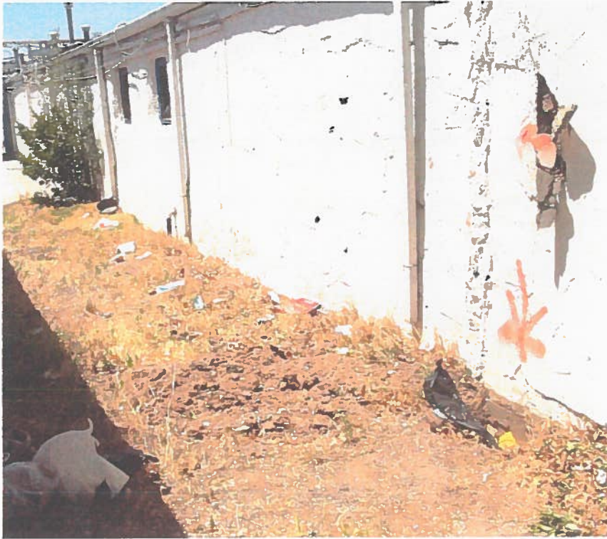
Figure 14 Soil Level Adjacent to Wall
