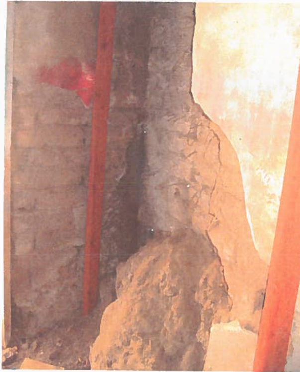
Figure 19 Collapsed Storage Shed Adobe Walls
