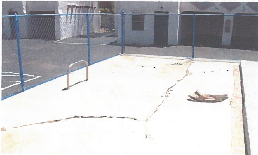
Figure 13 Cracked Concrete at Swimming Pool deck
