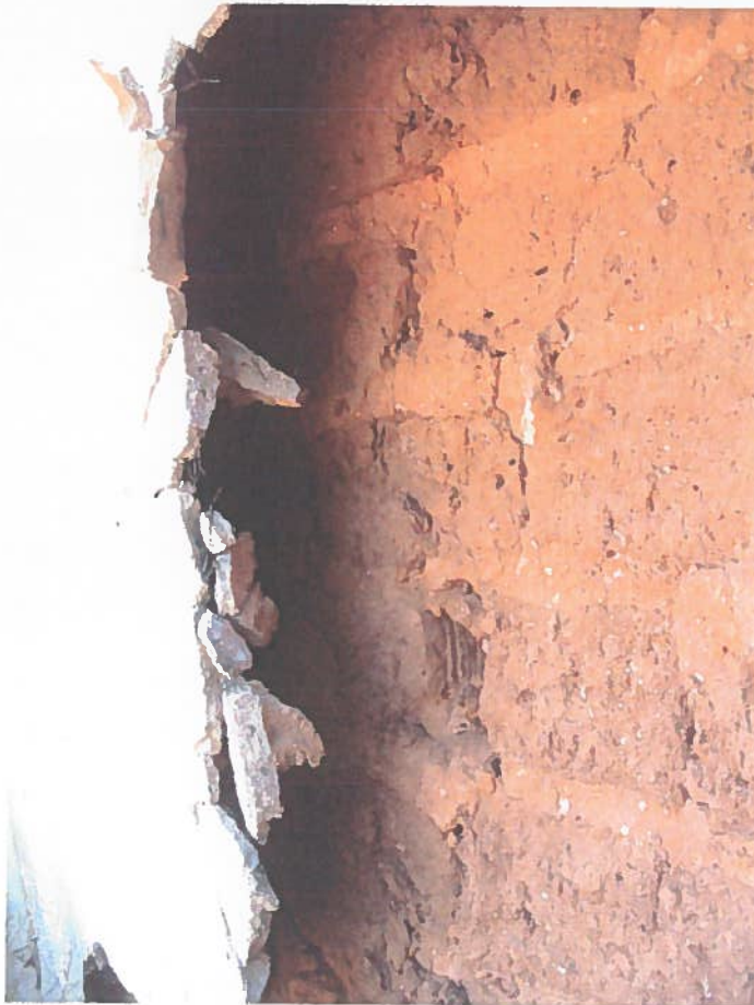
Figure 39 - Cement Stucco Separation from Adobe Wall
