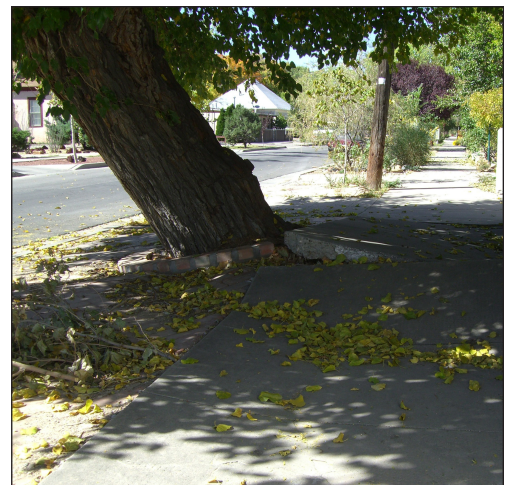
Sidewalk that has been buckled by tree roots
