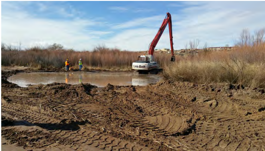
Excavation of the open water area at the San Antonio Oxbow, March 2016
