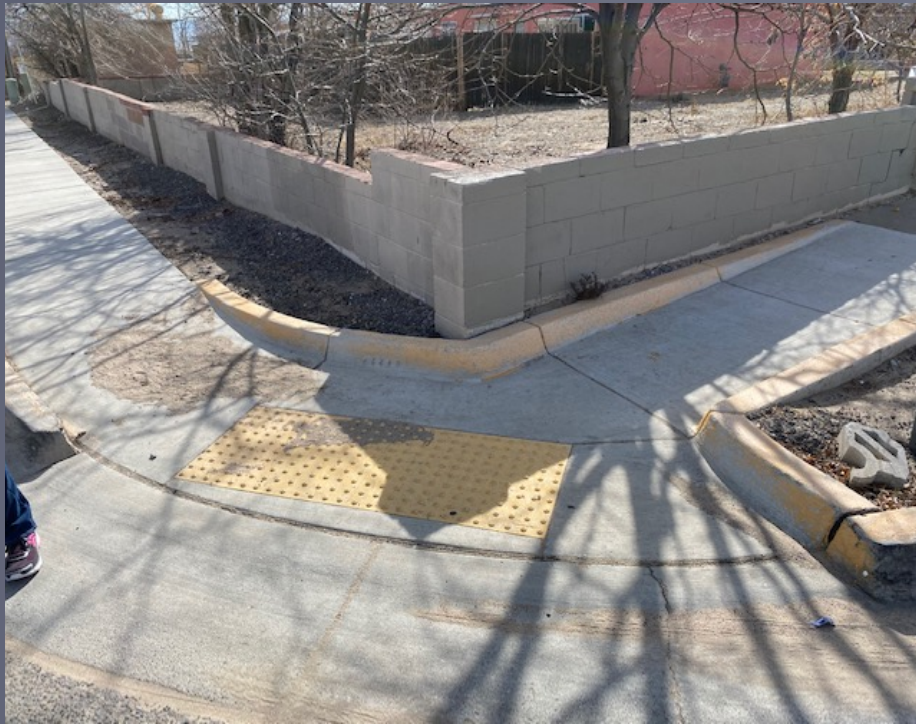
Non-Compliant Curb Access Ramps
