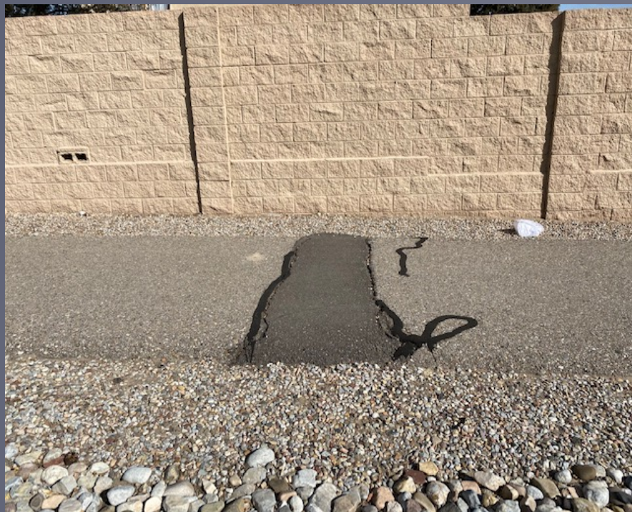
Poor Patchwork for Utility Crossings along Multi-Use Trail
