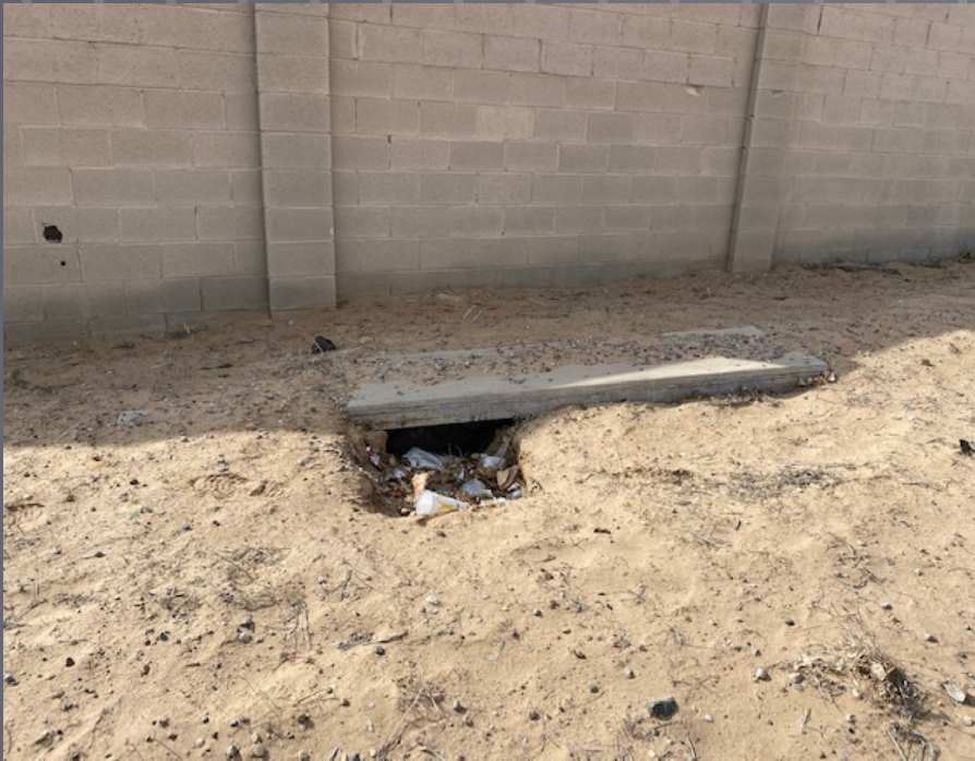
Incomplete Storm Drainage Infrastructure
