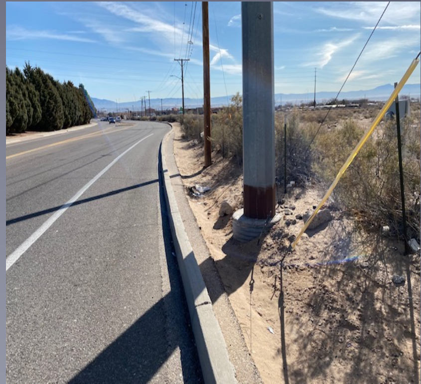
Inconsistent sidewalk along the south side of Devargas Road.
