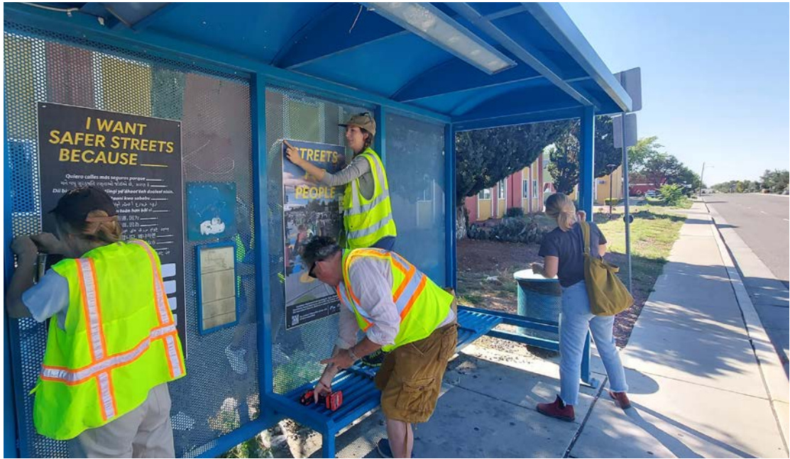
Installation of an interactive board at a bus shelter along Louisiana Blvd.
