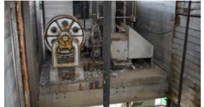
Mezzanine elevator machine room (cab has been removed).
