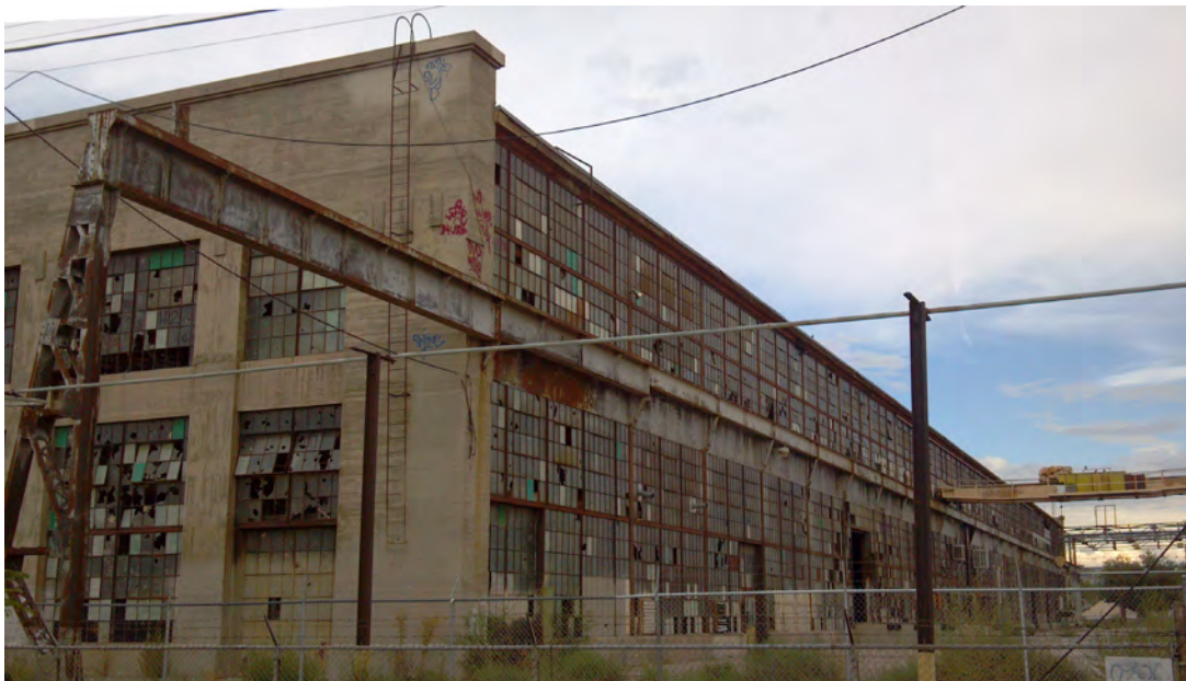
Current condition of Rail Yards buildings characterized by vandalism, graffiti and general neglect.
