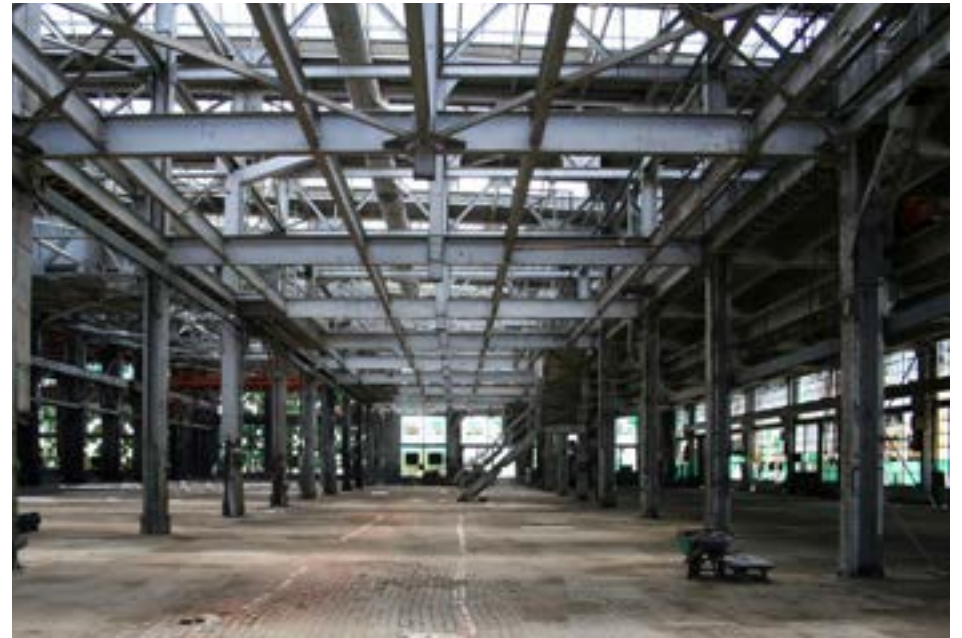
Machine Shop, light machinery bay, pyramidal skylights run between the heavy and light machinery bays.
