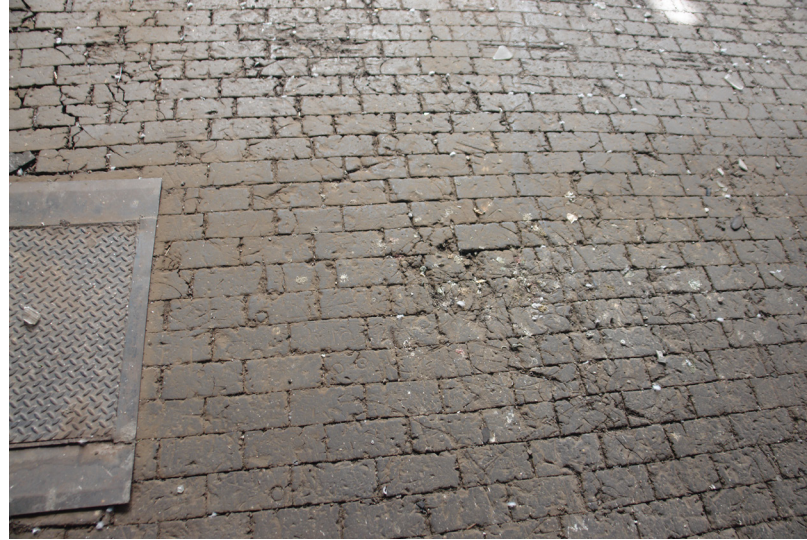
Machine Shop floor, 3" thick Kreolite creosoted woods blocks sit on a 6" thick concrete floor to dampen sound.
