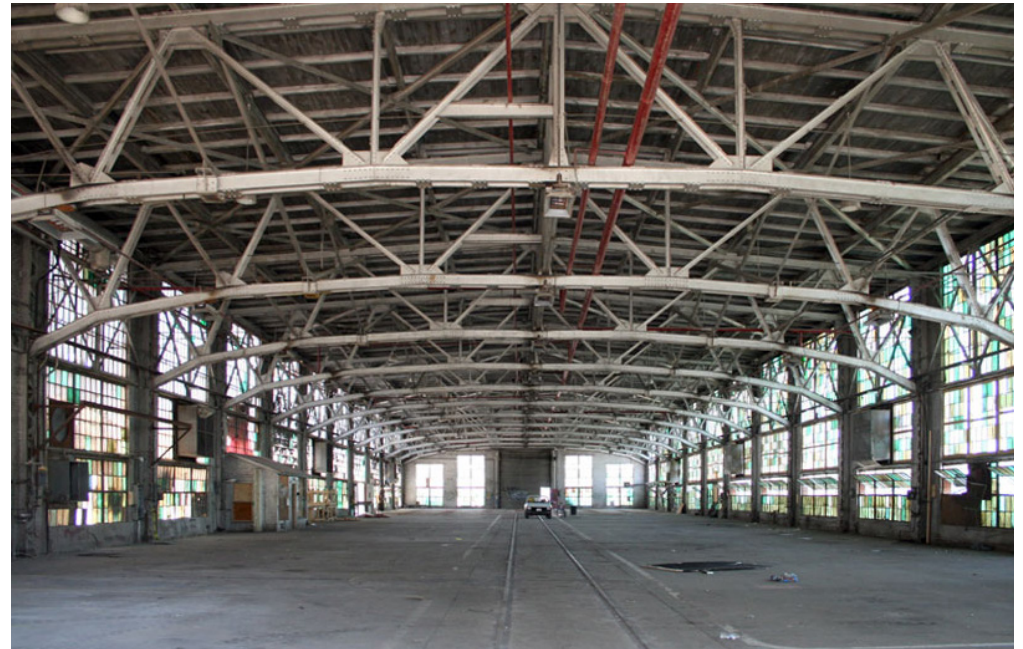
Blacksmith Shop, steel trusses, wood plank ceiling, glazed east and west elevations.
