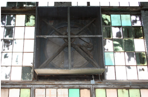
Fan equipment at glazed elevation.
