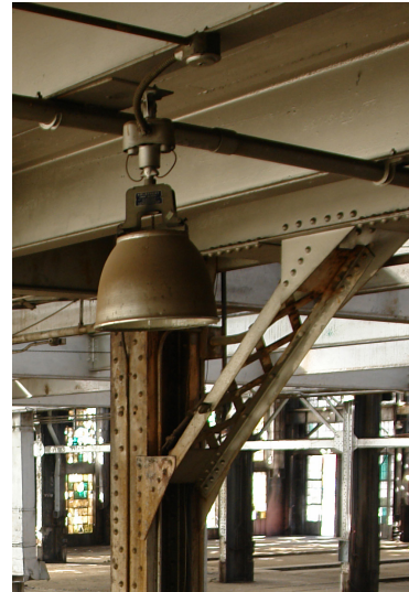
Machine Shop, existing high bay lighting.
