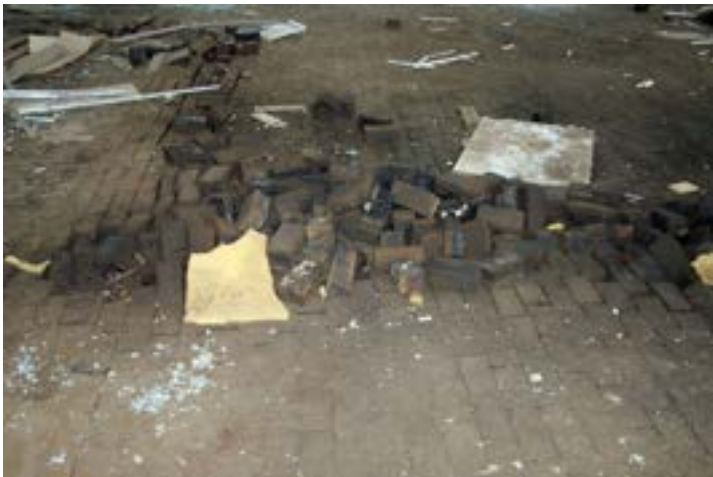
Damaged flooring, 3" thick creosoted end-grain wood blocks
