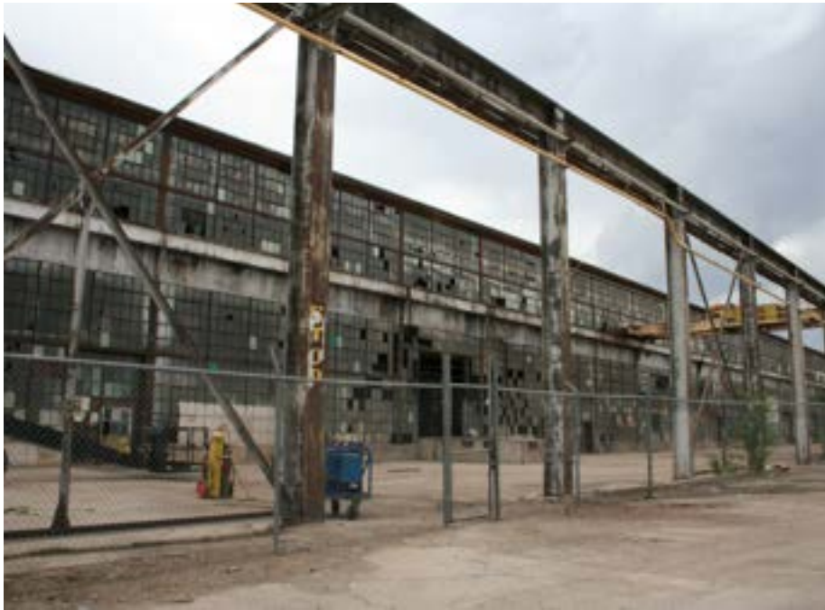
Bridge crane, view from southwest corner.
