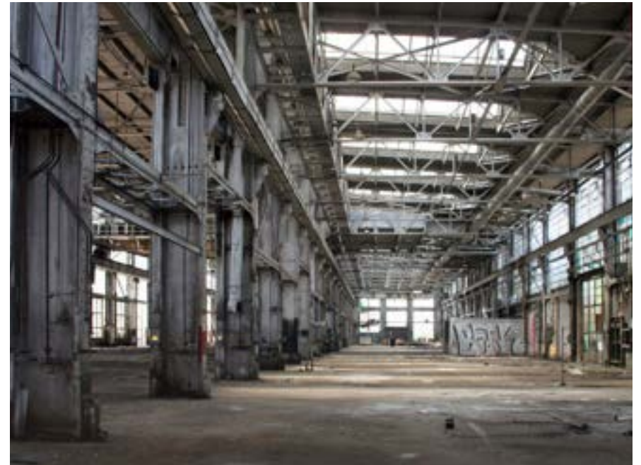
Boiler Shop, heavy equipment bay, pyramidal skylights, entrance to Flue Shop at immediate right.
