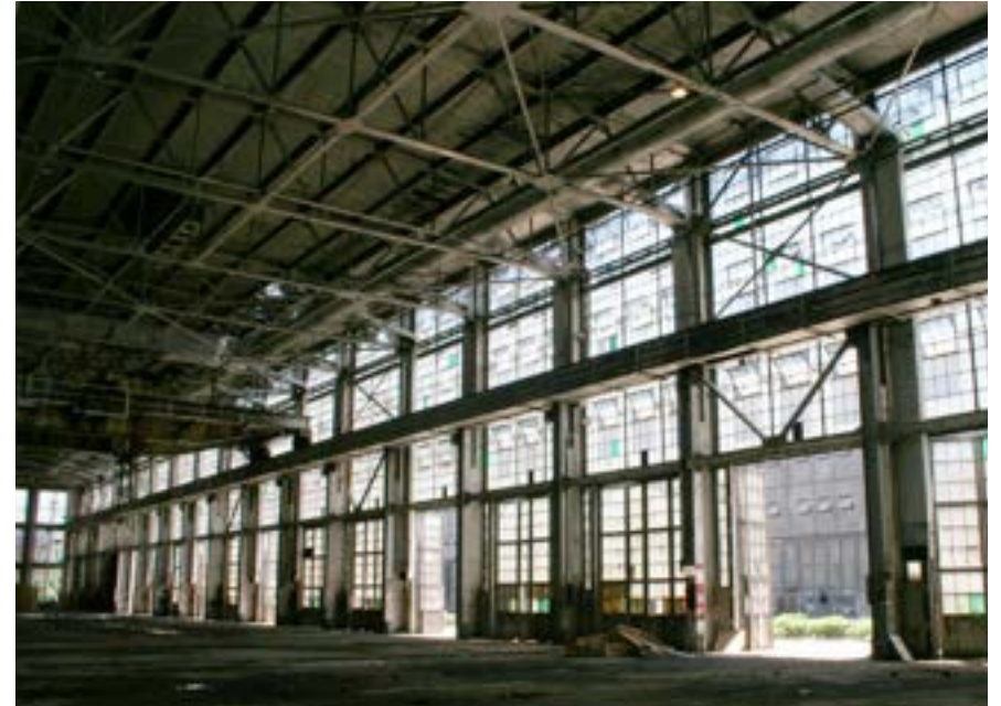
Boiler Shop, erecting bay, fully glazed southern elevation with 18' tall operable doors.
