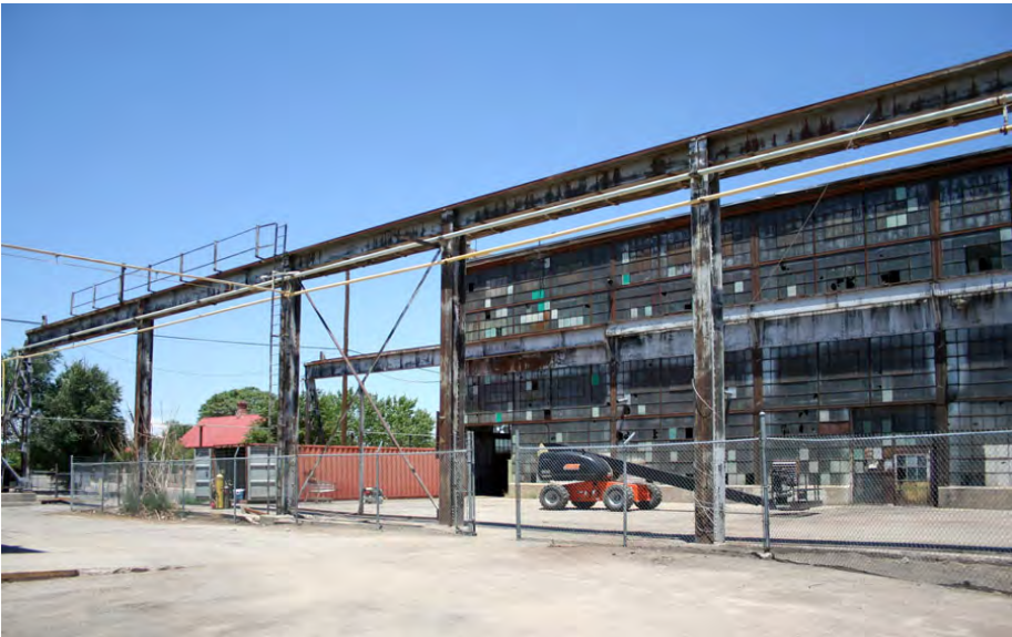
South bay, crane runway, exterior loading crane.
