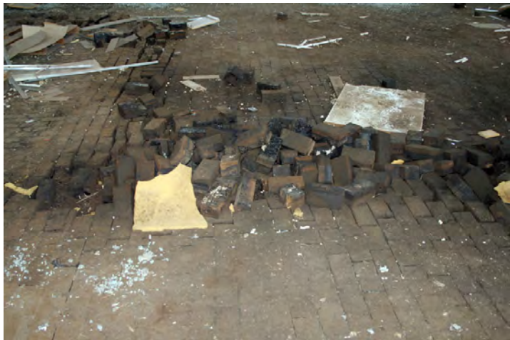
Damaged flooring, 3" thick creosoted end-grain wood blocks
