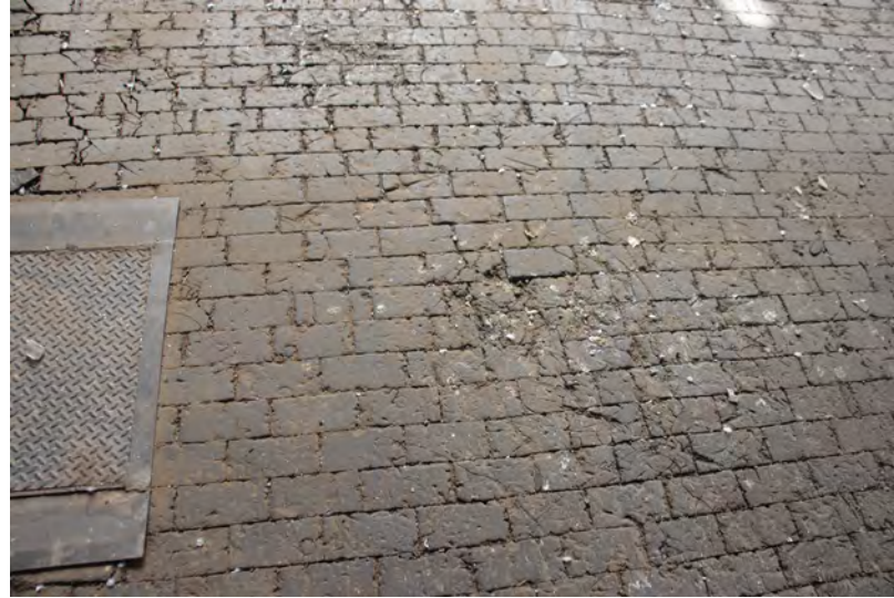
Machine Shop floor, 3" thick Kreolite creosoted woods blocks sit on a 6" thick concrete floor to dampen sound.
