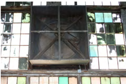
Fan equipment at glazed elevation.
