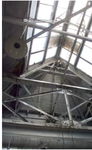
Gear/pulley mechanism for skylight operation.
