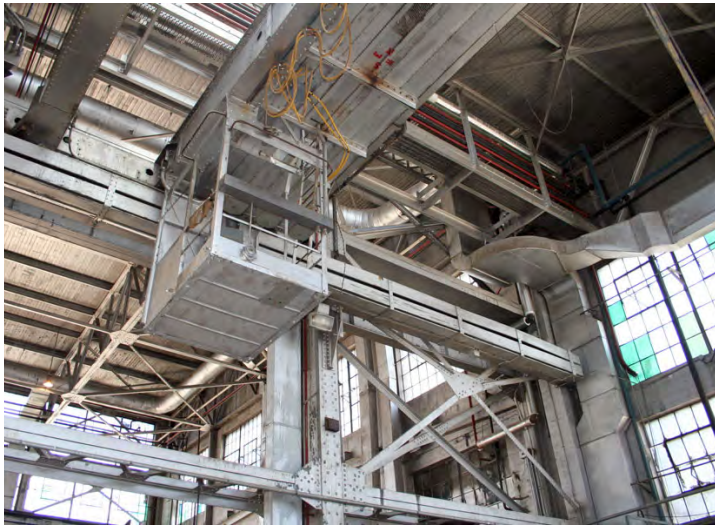
Crane operator workstation, heavy equipment bay.
