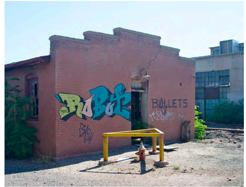
Condition of Rail Yards buildings characterized by vandalism, graffiti, and general neglect (2014).
