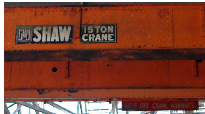
Machine Shop Crane specification/signage.
