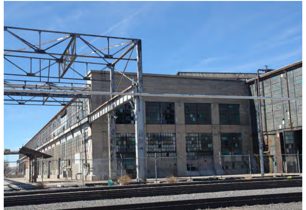
Bridge crane, view from east elevation.
