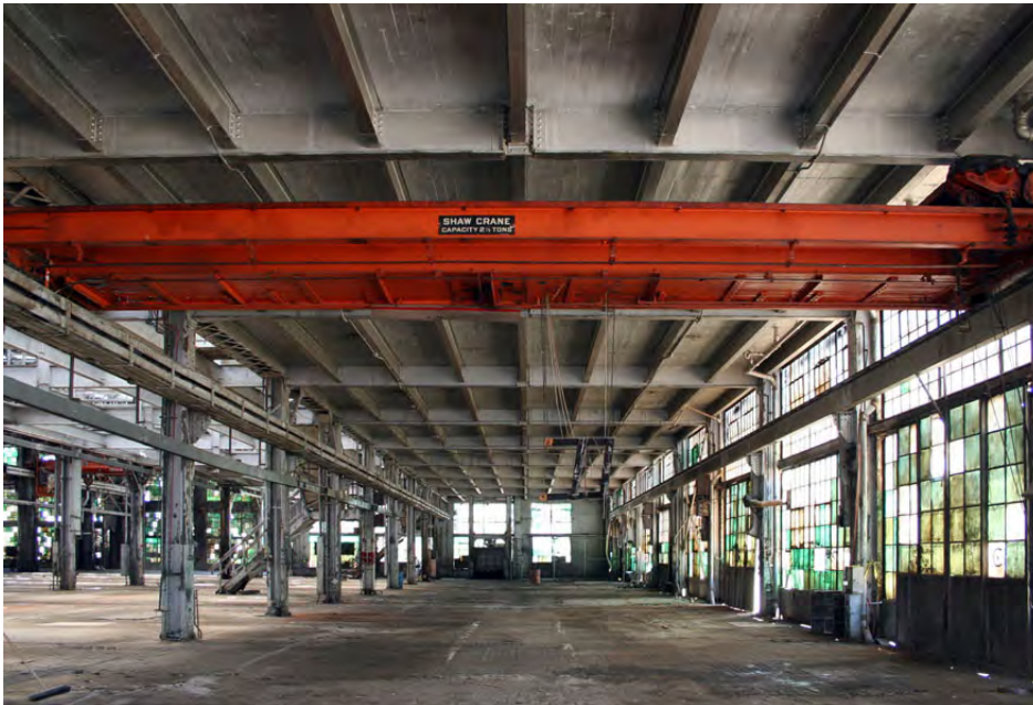
Machine Shop, bench bay - Below board formed, cast in place, concrete mezzanine.
