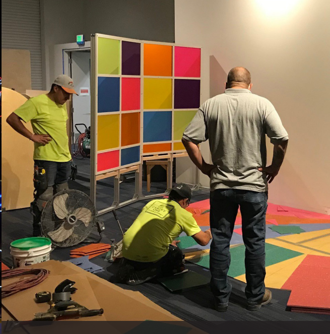
Elevation Station – The Balloon Museum’s Elevation Station was completed in 2020 and is ready to welcome visitors safely.
