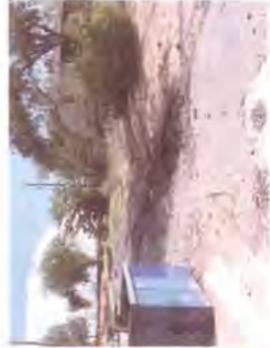
Drainage Problem, Apartments on the North-West corner of Ash and Buena Vista
